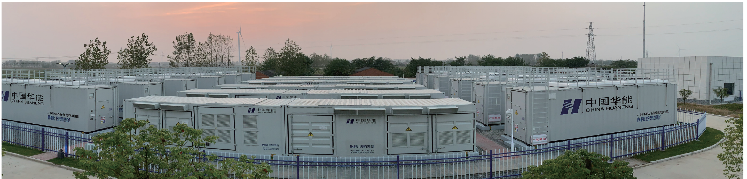
30MW/30MWh Huaneng Xiaojian Wind Farm Lithium Battery Energy Storage Project (EPC) Mengcheng, Anhui Province
