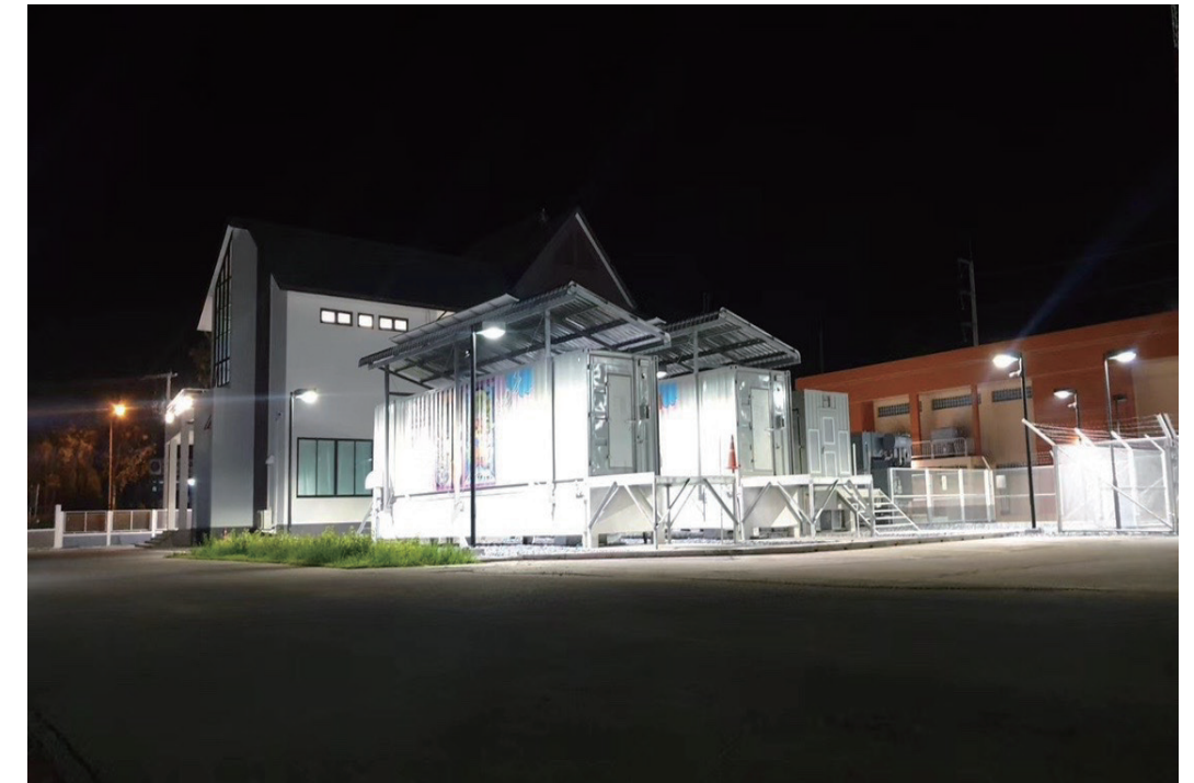
3MW/2MWh PEA Micro-grid Energy Storage Project , Thailand Micro-grid coordination control, auxiliary frequency regulation and voltage regulation
