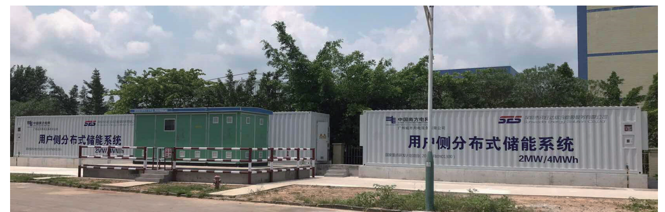
2MW/4MWh User side lithium battery energy storage project, Conghua, Guangdong
