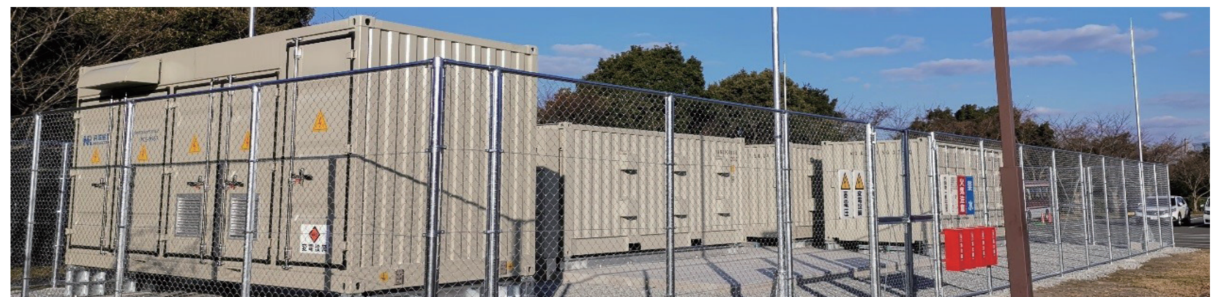
600kW/3.6MWh TOTO factory user-side sodium-sulfur battery energy storage project, Japan Auxiliary Services, Power Tracking
