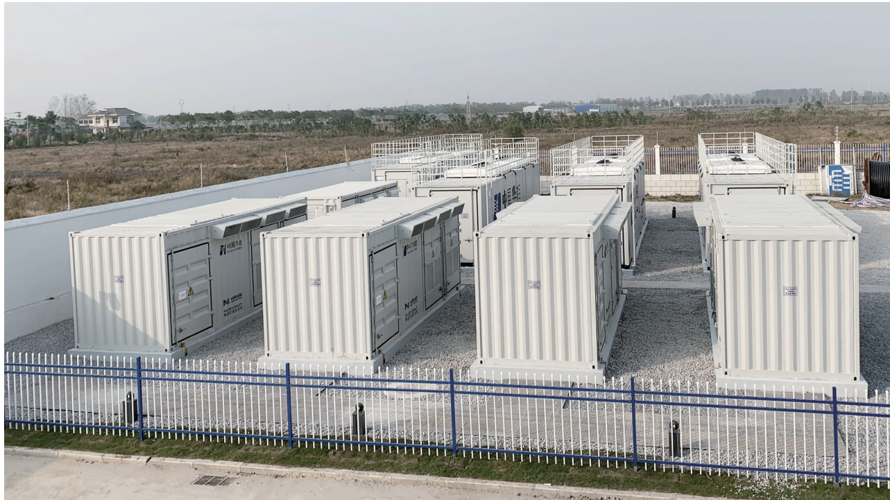
10MW/10MWh Huaneng Xutuan Wind Farm Lithium Battery Energy Storage Project (EPC) Mengcheng, Anhui Province
