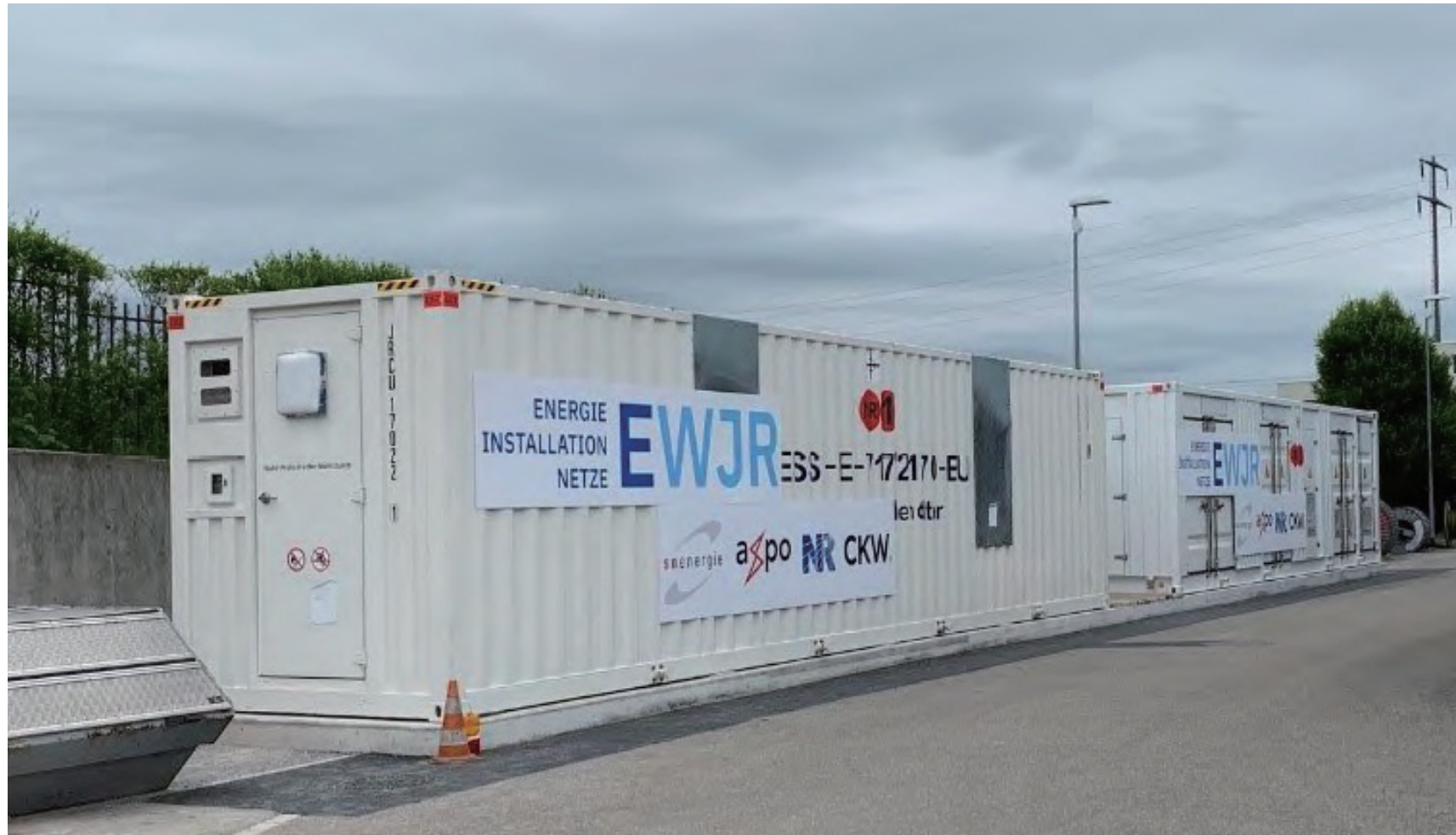
2MW/2.17MWh EWJR lithium battery energy storage project , Switzerland Power grid peak shaving, frequency regulation and voltage regulation
