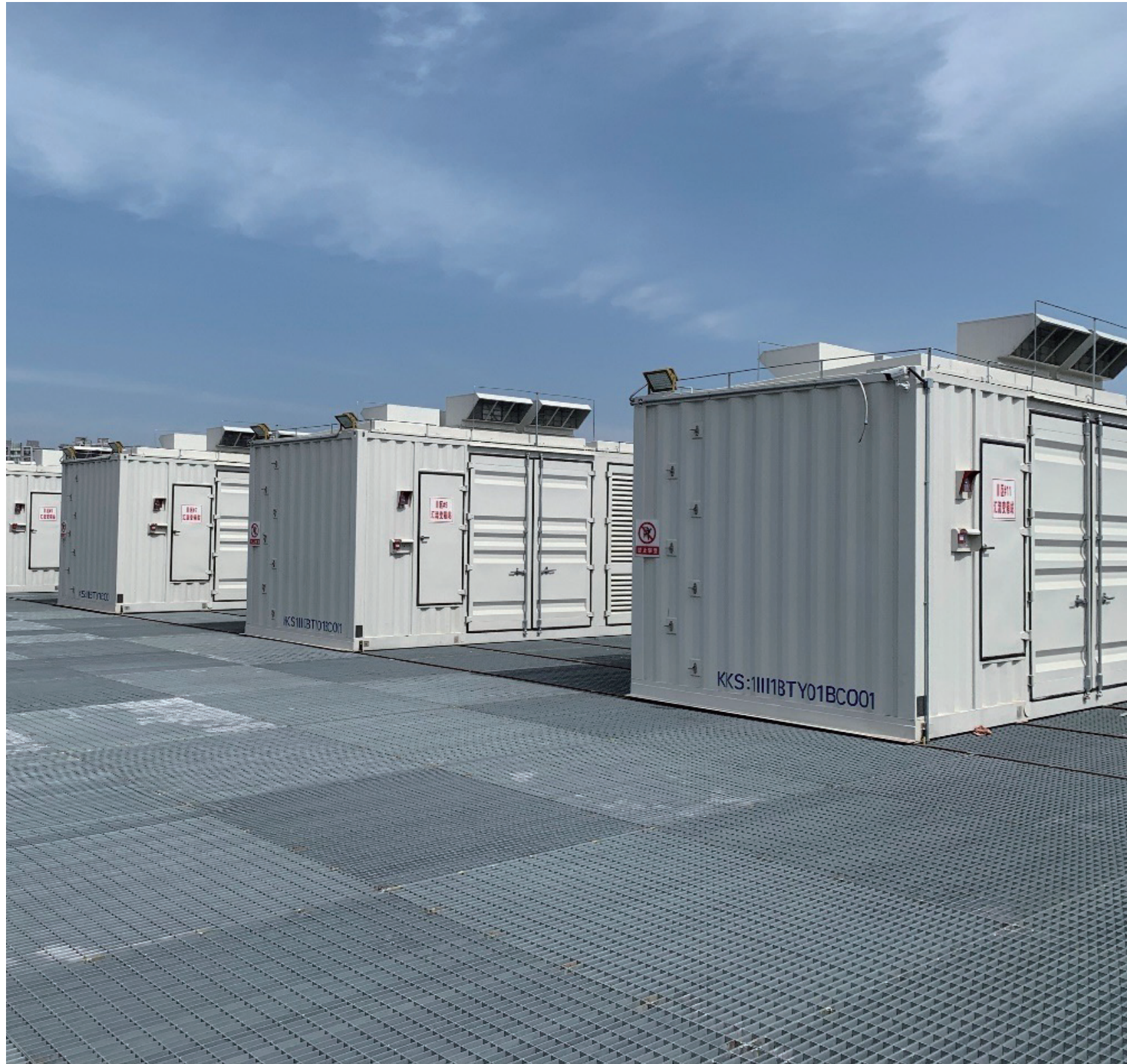
100MW/400MWh Vanadium-redox-flow-battery Energy Storage (PCS+PMS+EMS Integrated Supply) Dalian, Liaoning
