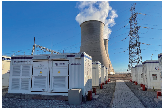
10MW/5MWh Zhangye Power Plant Energy Storage Frequency Regulation Project Zhangye, Gansu
