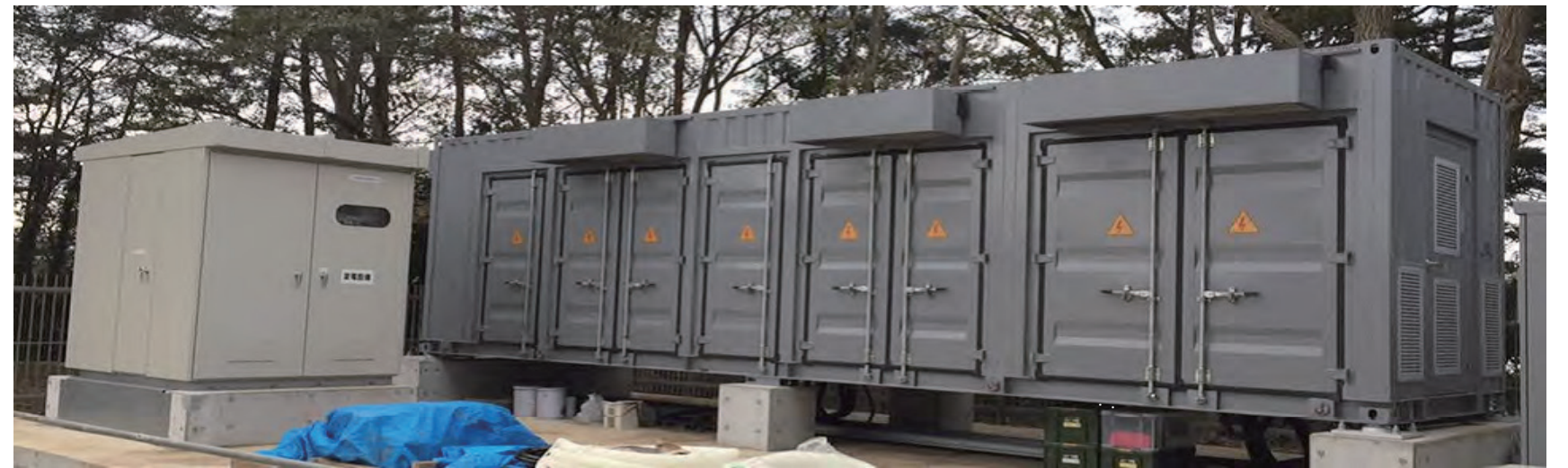
1MW/2MWh Ibaraki user-side Vanadium Redox Flow Battery energy storage project, Japan Peak shaving and valley filling, off-grid main power supply
