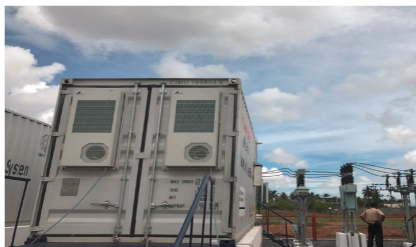
1MW/0.5MWh India Power Grid first energy storage system, India Peak shaving and valley filling, auxiliary frequency regulation
