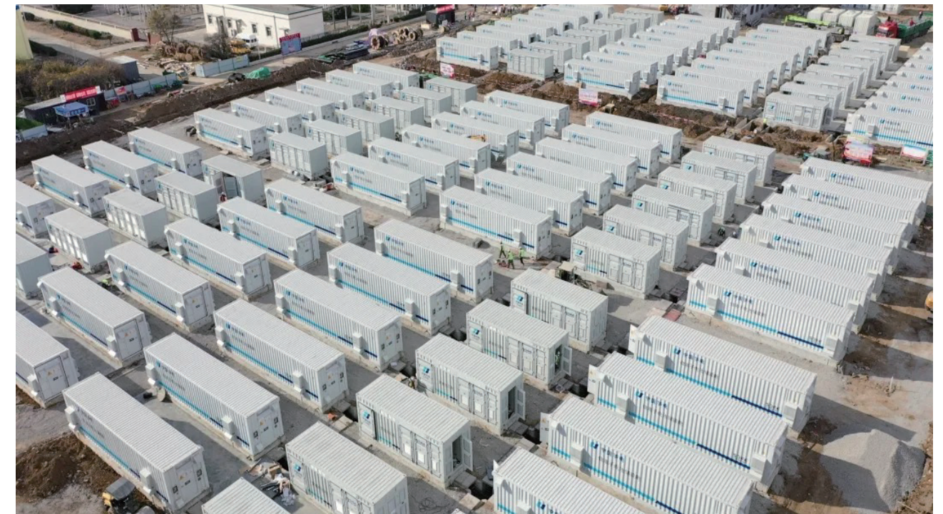
101MW/202MWh Huadian Tengzhou Power Plant Peak Shaving Energy Storage Project (PCS+PMS+EMS integrated supply) Tengzhou, Shandong
